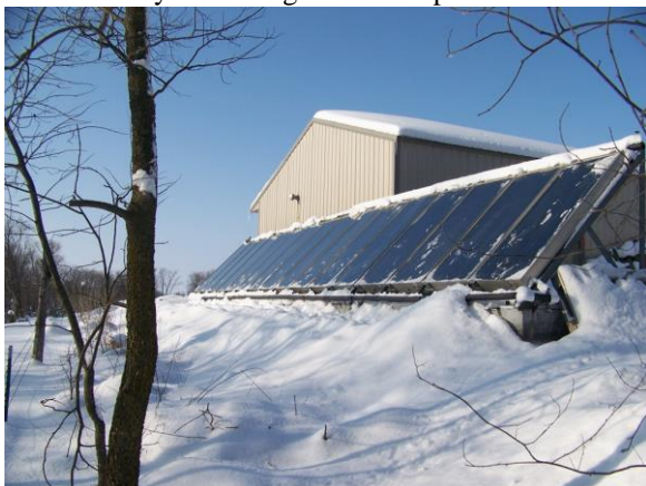
Figure 2.1. Solar panels in Germany
